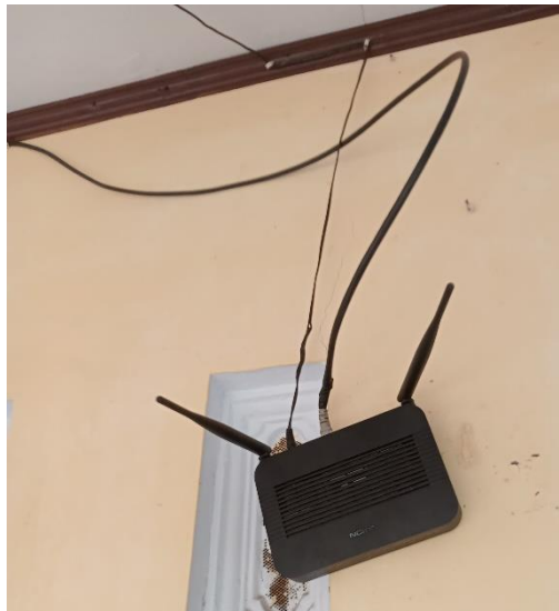
Figure 5. First point Router Signal
